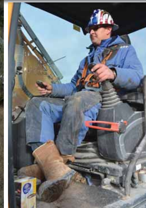
Above: Operator Klaas Brinkman usually works from ground level in the cab of a high-reach demo rig, and says top-down demolition is completely different.
