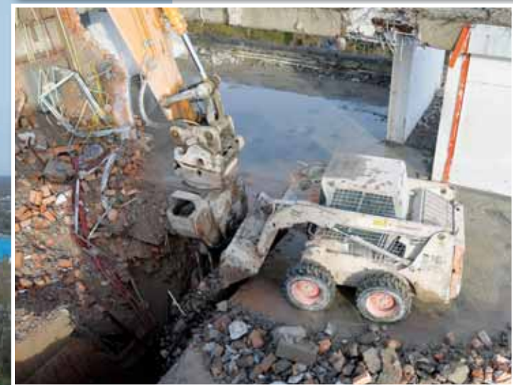
Above: Hoisted to the top, a Bobcat S160 shovels debris down the lift shaft to create a level surface to move the platforms down a floor.
